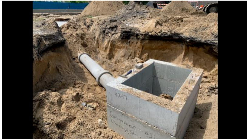
Figure 1: Grimmer Installed STR 247
